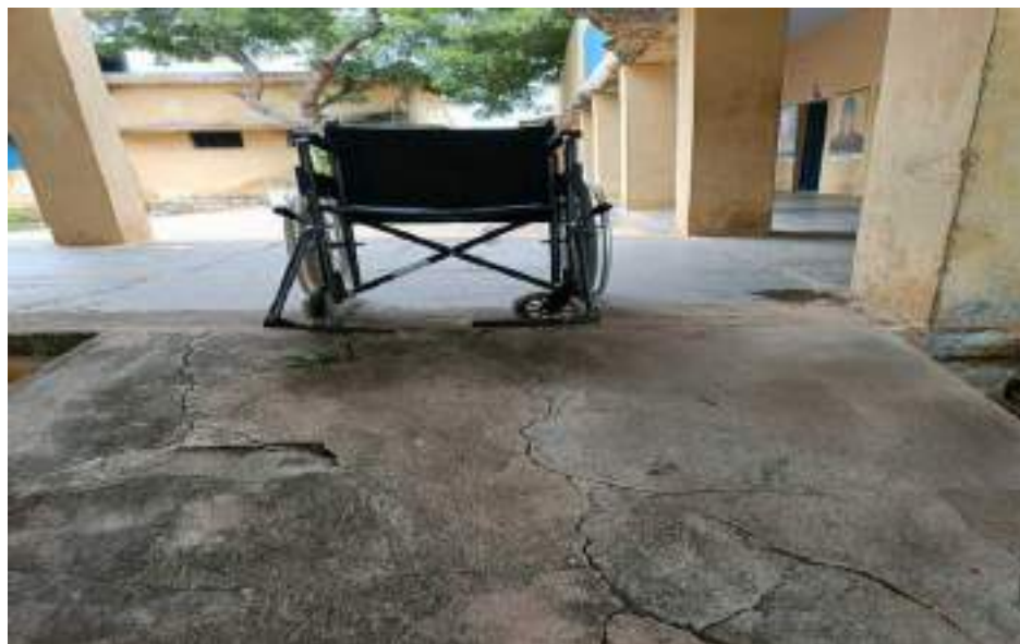
Ramps for disabled
